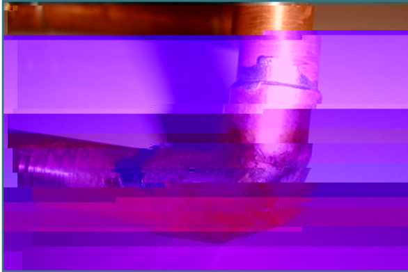
Copper pipes joined by lead solder.
